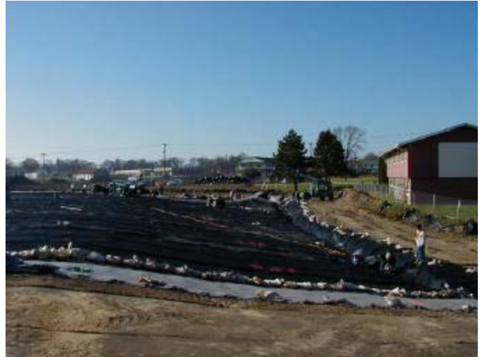
Construction of a RCRA-equivalent landfill cap on Landfills 6 and 7 at Fort Sheridan.
