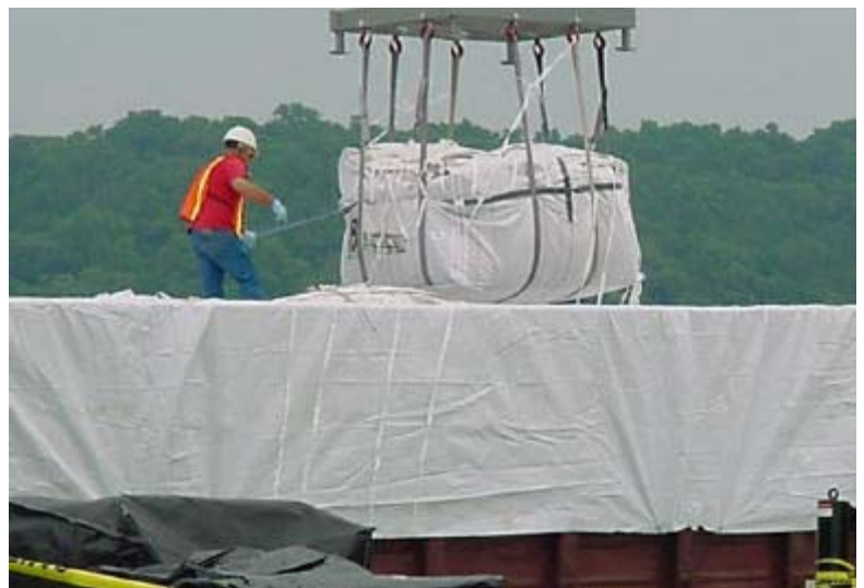
At Savanna Army Depot Activity, Army contractors transfer a container filled with pesticide to a rail car.
