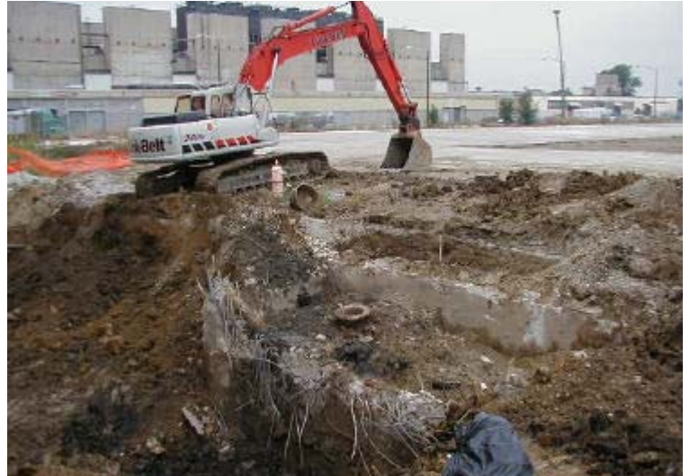
Previously undiscovered underground tanks were found in concrete vaults beneath railroad tracks at Air Force Plant #39.
