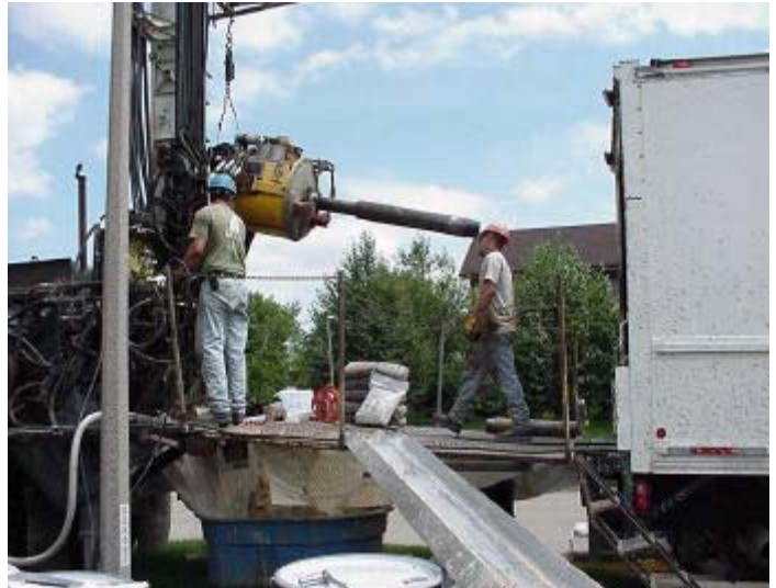
A sonic rotary drill rig being used to install monitoring wells at the former Nike Missile Battery Site C-70.
