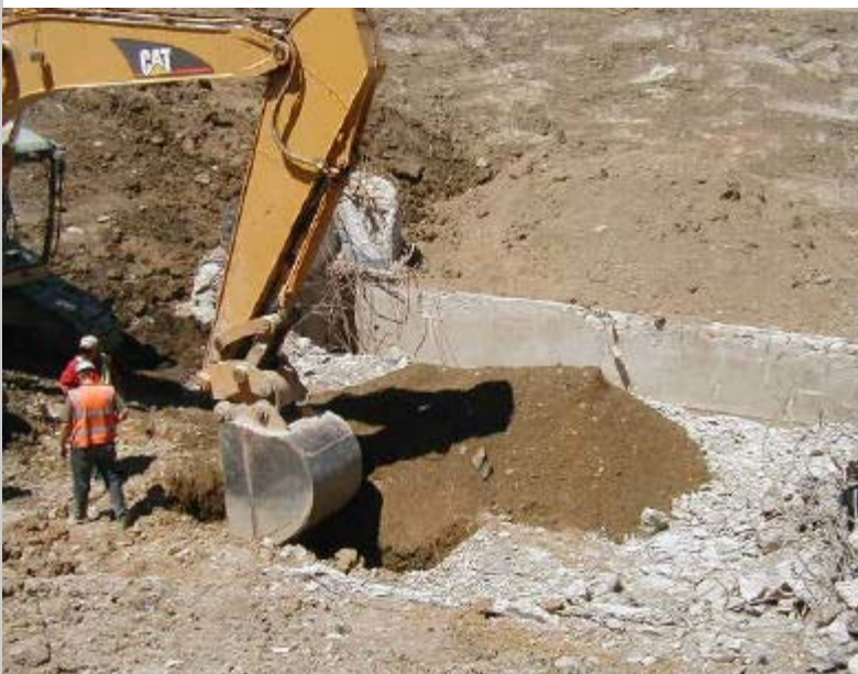
Navy contractors excavate fill material in the floor of a Nike missile magazine at the Libertyville Training Site.
