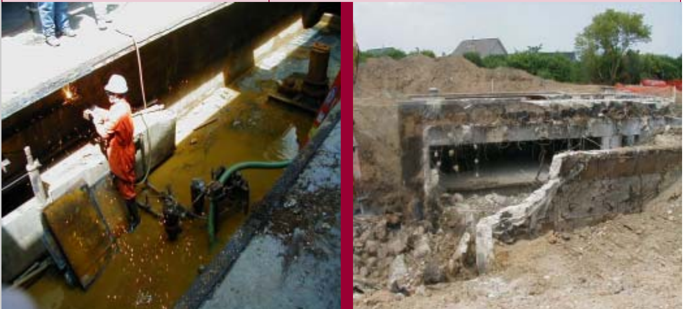
Demolition in progress at the Libertyville Training Site Nike Anti-aircraft Missile Batteries.
