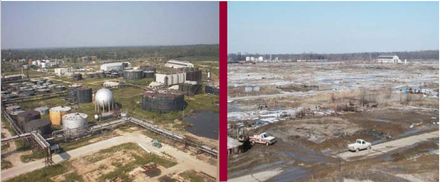
The Texaco/Indian Refining Company NPL site before and after site demolition (note the upper-left fabrication shop building in both photographs).
