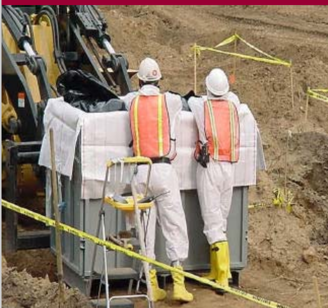
Removal of dinitro-ortho-cresol pesticide contamination at the Savanna Army Depot Activity NPL site.
