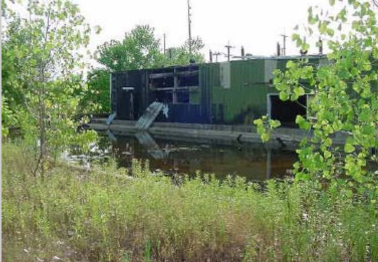
The former creosote tie treatment building and treatment basin at the Jennison-Wright NPL Site will be removed in FFY 2003.
