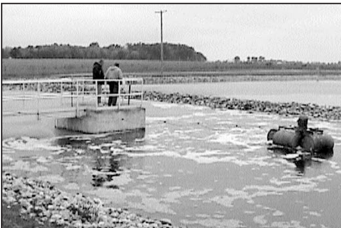
Rend Lake conservancy District, final lagoon cell transfer structure.
