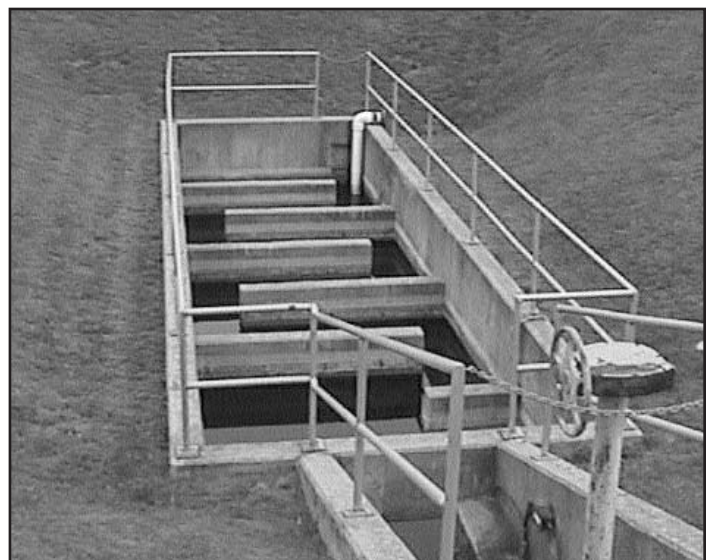
Breese chlorine tank.
