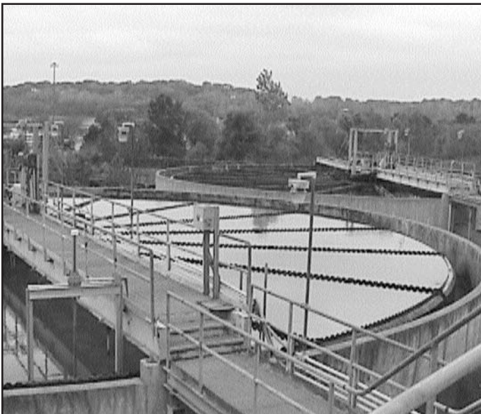
Caterpillar/Mapleton dust collector wastewater primary clarifier.
