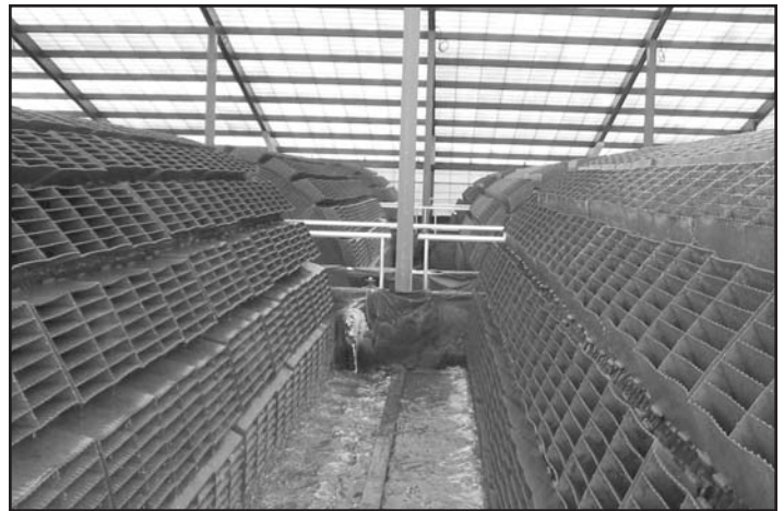
Covered RBC units at the Jerseyville wastewater treatment facility.
