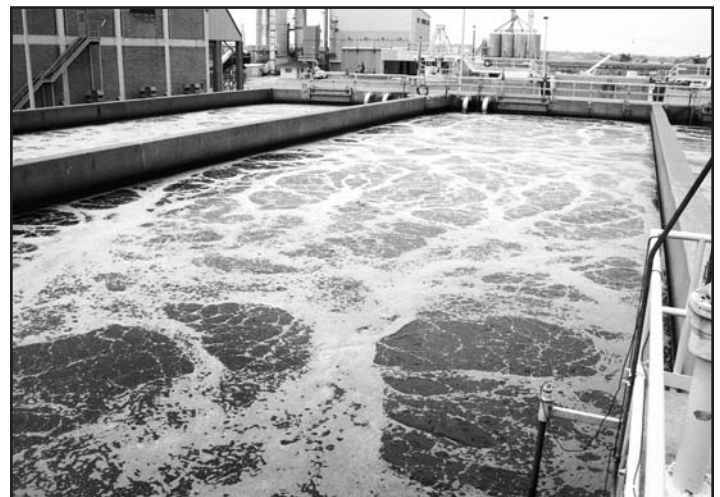
Wastewater treatment facility.
